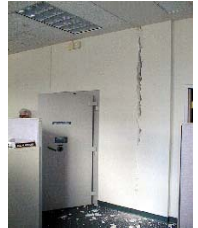
A walk-in safe in the insurance building showed signs of damage following the quake.
