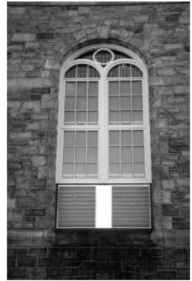
Pictured is one of the replacement windows at Rhode Island's historic maximum security prison in Cranston.
