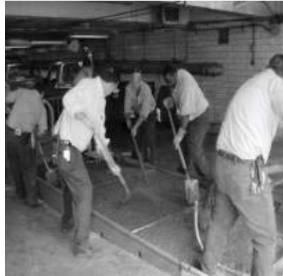
A GBA support team is shown pouring concrete to create a sturdier entrance in a parking garage.
